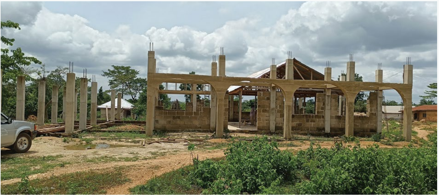
A new church building is being constructed in the Obuasi area of Kumasi, Ghana. It will be the largest church facility in the area and the only Adventist-believing church in the region.
